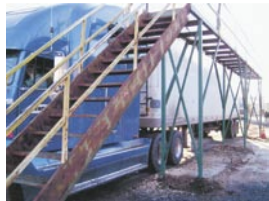
Fig. 3: Catwalk is approximately the same height as the top of the trailer. (South Carolina sawmill location)
